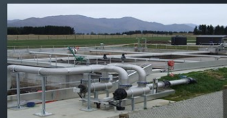
Treatment and disposal facilities
